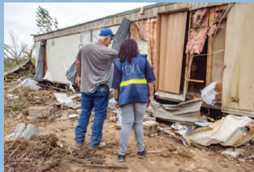
FEMA official assess TN storm damage
